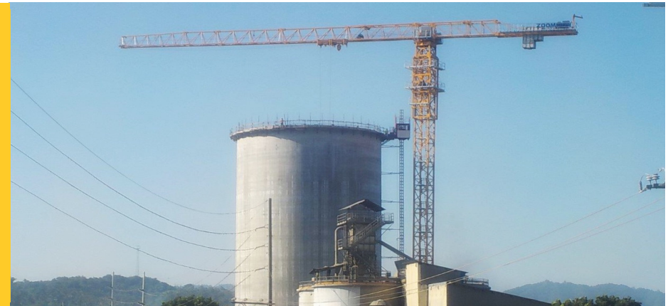
Republic Cement Iligan Inc. are increasing the cement production capacity at their Iligan Plant. BEC was appointed as the contractor for construction of the dual cell silo.
