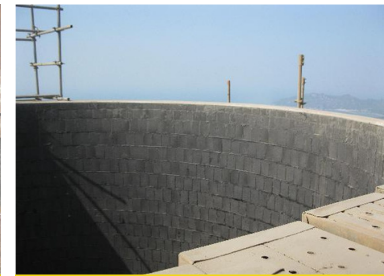
Completed installation of Pennguard Borosilicate Blocks at the top of the flue
