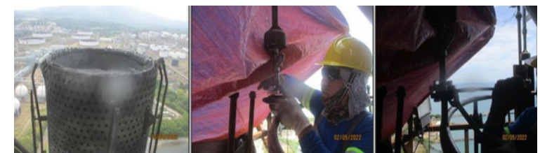
Repair and installation of all eight (8) pilot tips of the acid flare tip.
